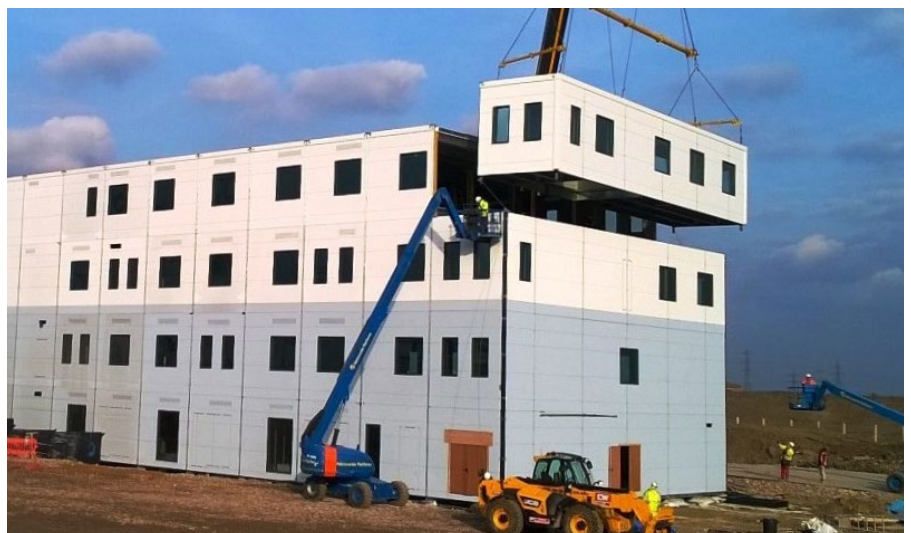
Example of modular construction: The London Borough of Barking and Dagenham - Riverside Campus. Modular construction allowed 23,800m 2 to be constructed in 19 months.
